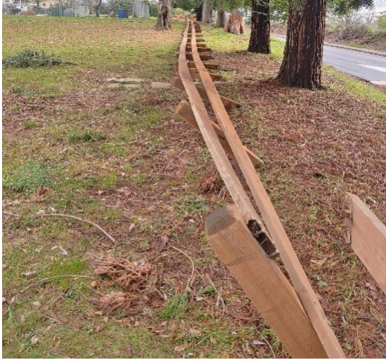
Figure 1. Fallen fence at the Aquatic Park after it fell during the last storm.
