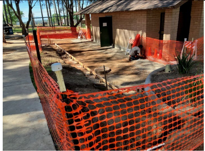
Figure 6. The maintenance crew is doing more work to make Bille Park ADA accessible.
