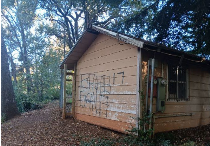
Figure 1. Vandalism on the Aquatic Park shed before.
