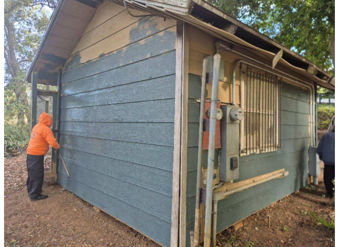
Figure 2. Vandalism on the Aquatic Park shed after.
