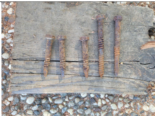
Figure 3. The old bolts used to hold the bridge together at the Aquatic Park.
