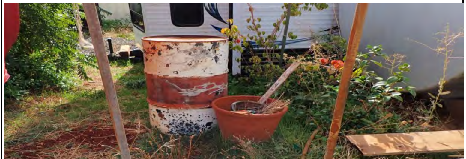
Image 9. View of rusted tank and additional materials.
