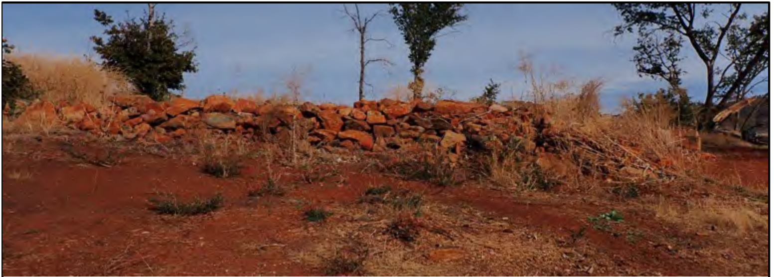
Image 40. Stacked pile of rocks, concrete and dirt in the footprint of a second former structure.
