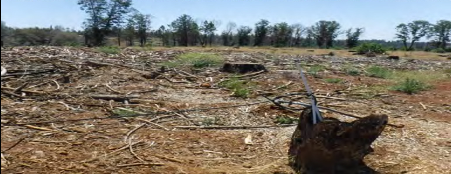
SITE PHOTOGRAPHS – JUNE 7, 2021 LAKERIDGE PARK PROJECT EAST OF LAKERIDGE CIRCLE AND WEST OF DOGTOWN RD, MAGALIA, CA
