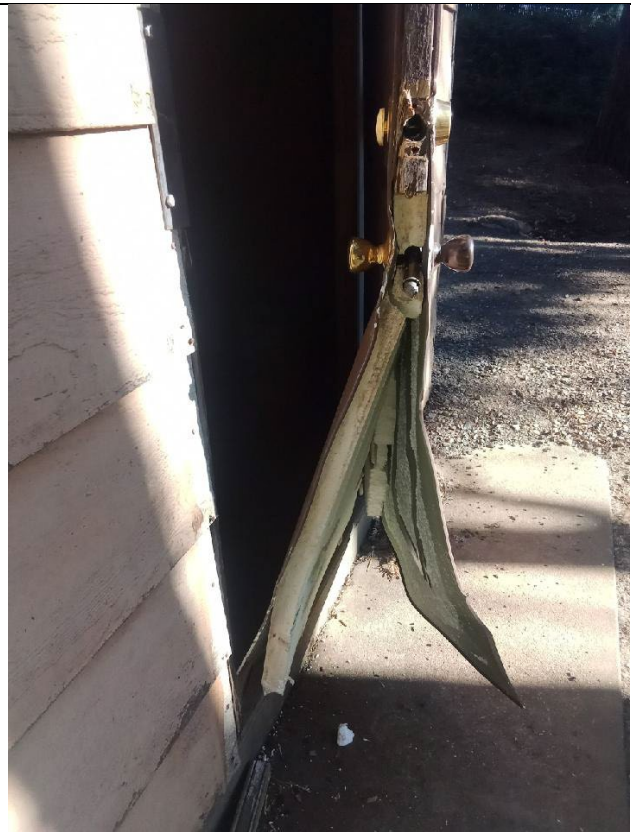
Figure 7. Damaged pump house door at Aquatic Park.
