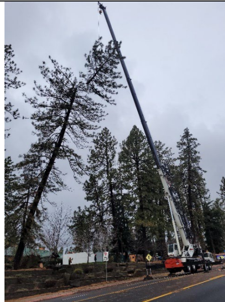
Figure 8. Mark D Cobb, Mike Houdek and D.J. Gomes (owner of Crossfire Tree & Vegetation Services), worked together to safely remove the tree before it fell onto the Skyway.
