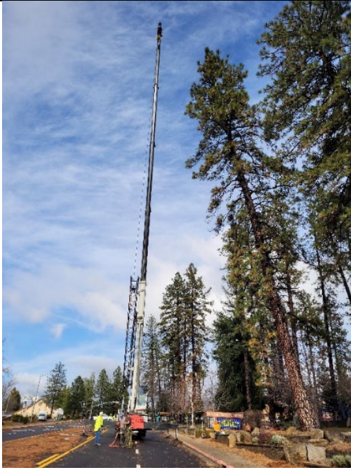
Figure 9. Mark D Cobb, Mike Houdek, and D.J. Gomes (owner of Crossfire Tree & Vegetation Services), worked together to safely remove the tree before it fell onto the Skyway.
